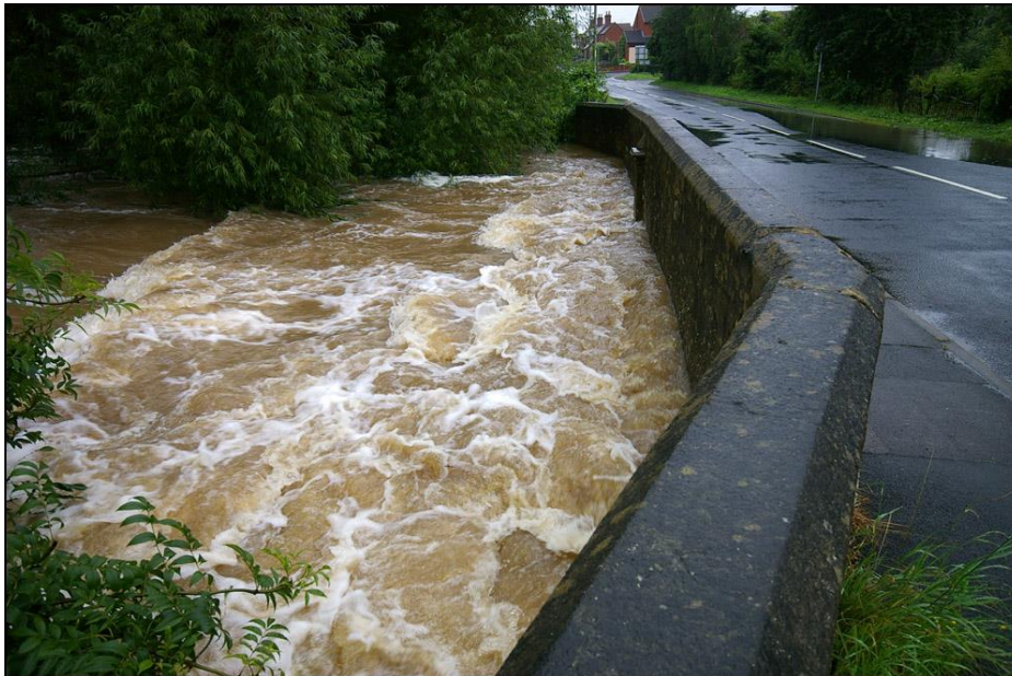
FIGURE 1.1 : Wyre Bridge during 2007 flood event
