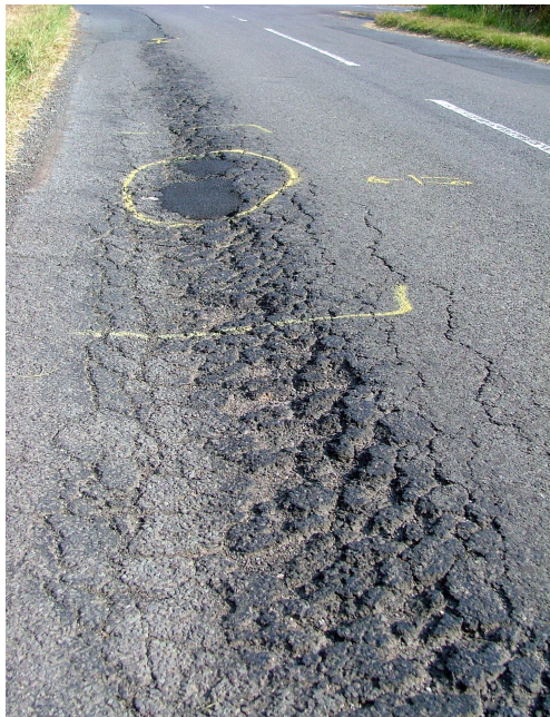
Photo 5: Deteriorating road surfaces
