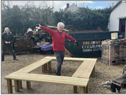
Photos: Various stages of construction and final product to prove weight-bearing capabilities!
