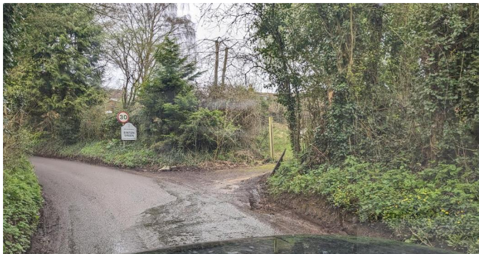
Image above shows water coming out of the Severn Trent facility and shows the eroded road surface.
