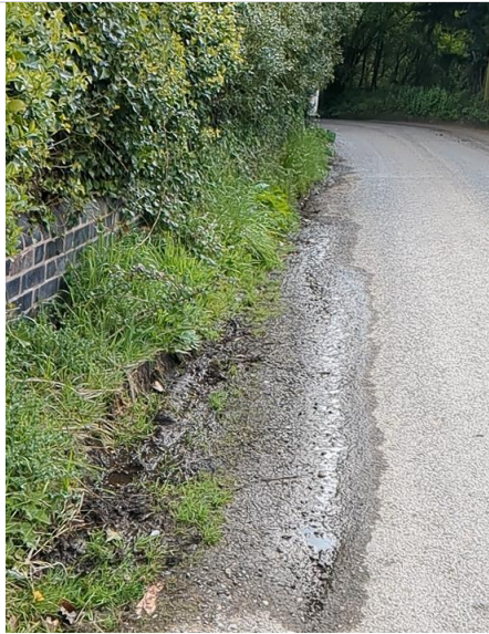
Image above shows water bubbling up through road outside Primrose Cottage, Dark lane, Sinton Green.
